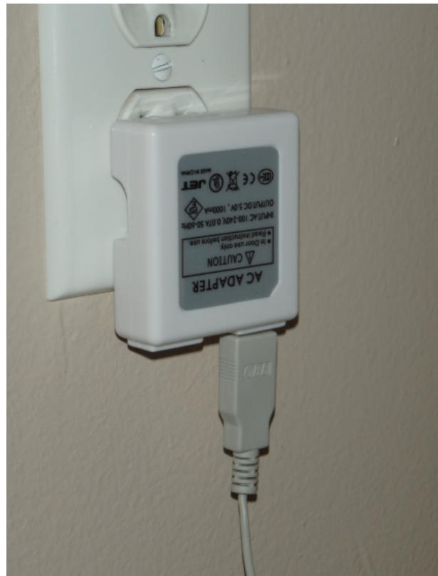
ACpower Charger in Use
